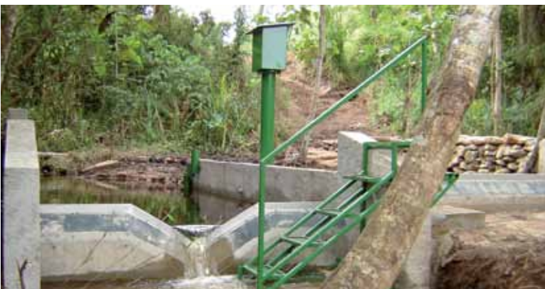
Hydrological Monitoring Station in Igaratá
